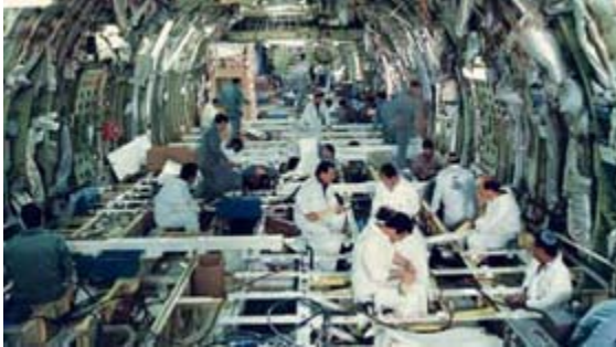
Picture shows Bedek engineers working on the floor beam replacement of a B747.
